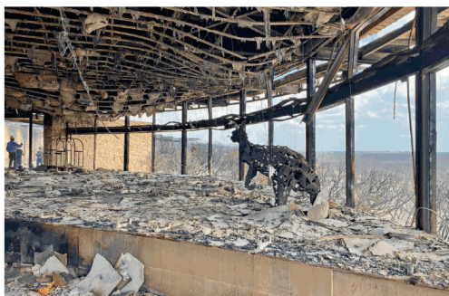
Above: the original Southern Ocean Lodge after the January 2020 fires. “From the moment it burnt down, I was absolutely hell-bent on rebuilding it,” Hayley Baillie says.
